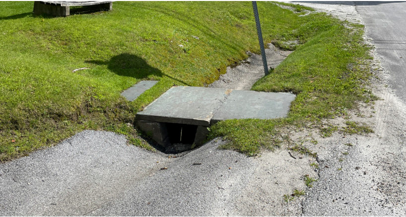
Stormwater Inlet. Open stormwater inlet interferes with on-street parking potential and can be a hazard for pedestrians.
