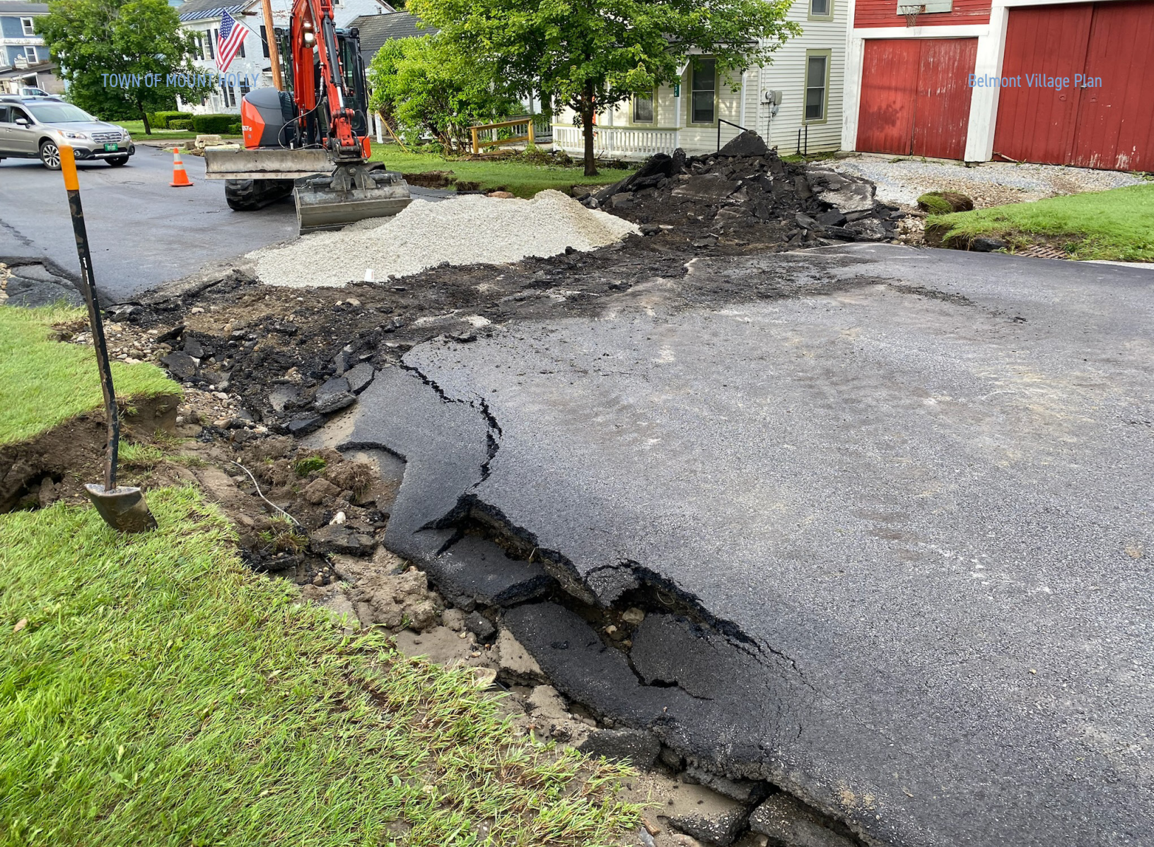
July 9, 2023 Storm Damage. Damage and repairs underway at Belmont Road, where the surcharging culvert compromised the road integrity (above); Photo inside the existing culvert where structural damage and failure is clearly visible (below).
